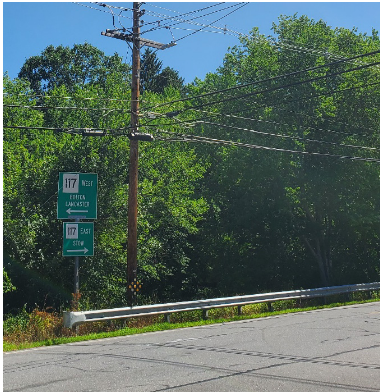
Figure 5: Existing guardrail with lack of reflective markers for visibility and faded object marker.
