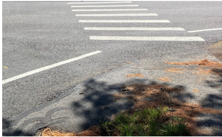
Figure 4: Non-compliant curb ramp on the southwest corner of the study intersection.
