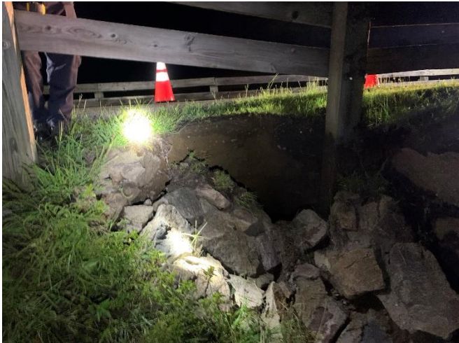
Figure 2: Photograph of sinkhole showing collapsed layer of grouted riprap and guardrail post falling into hole.
