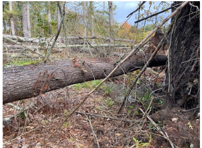
Figure 8: Another view of uprooting of pine trees along the downstream dam embankment. The trees and their roots will be removed.
