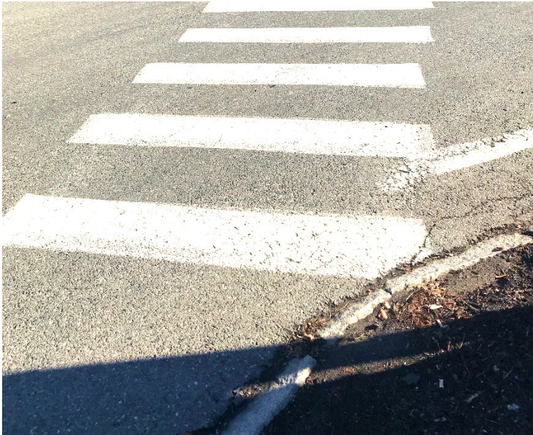
Figure 13 Lack of Pedestrian Facilities on Southwest Intersection Corner leading to Gleasondale Road (Route 62) Crosswalk
