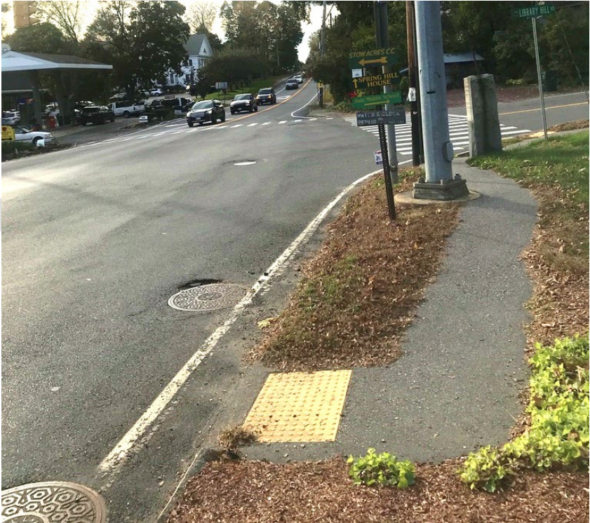
Figure 6 Great Road (Route 117 and 62) Crossing on Northeast Intersection Corner with Pedestrian Detectable Warning Strip Lacking Crosswalk
