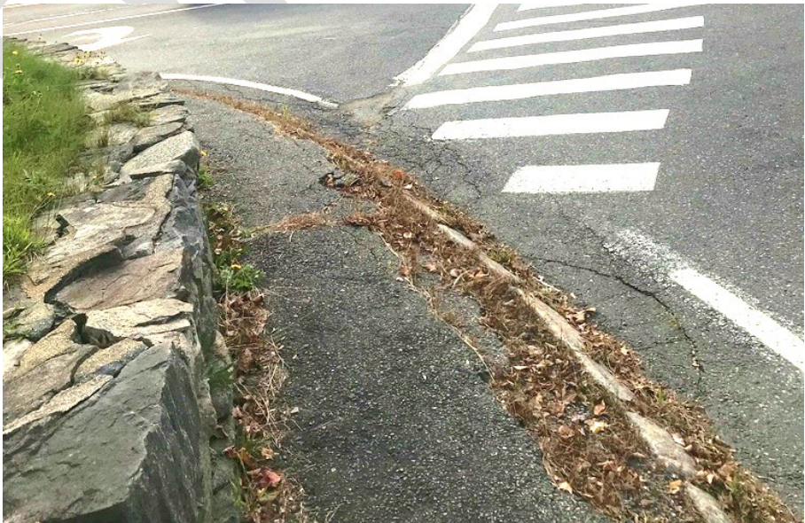
Figure 16 Southeast Intersection Corner Crosswalk Lacking Pedestrian Facilities
