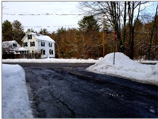
Packard Road in poor condition, facing Boxboro Road.
