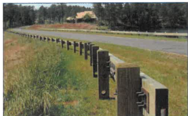
Figure 2: Example of steel-backed timber guardrails.
